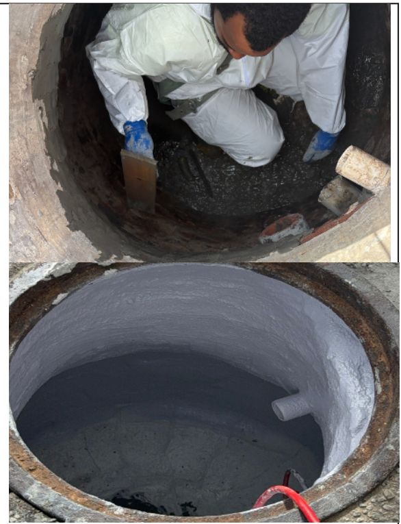
Top: Application of Mortartec Silicate to fill mortar joints and create a smooth, uniform substrate for subsequent protective coatings.
