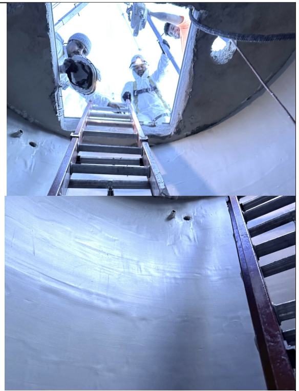
Above: Southern Painting & Maintenance Specialist looking into the completed wet well application.
