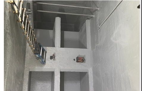
Above: Lift station lined and protected using Epoxytec's CPP Sprayliner (Summit Twp., Jackson County, MI)
